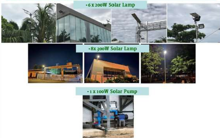
Use of solar lights in Mandaue Terminal
