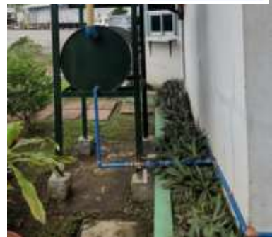
Tacloban Terminal's rainwater harvesting set-up
